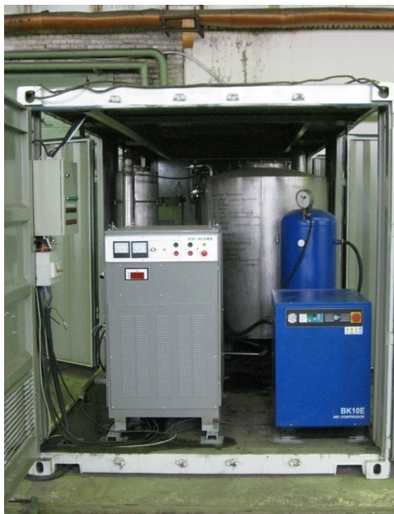
Figure 2: Power supply system and air compressor.
